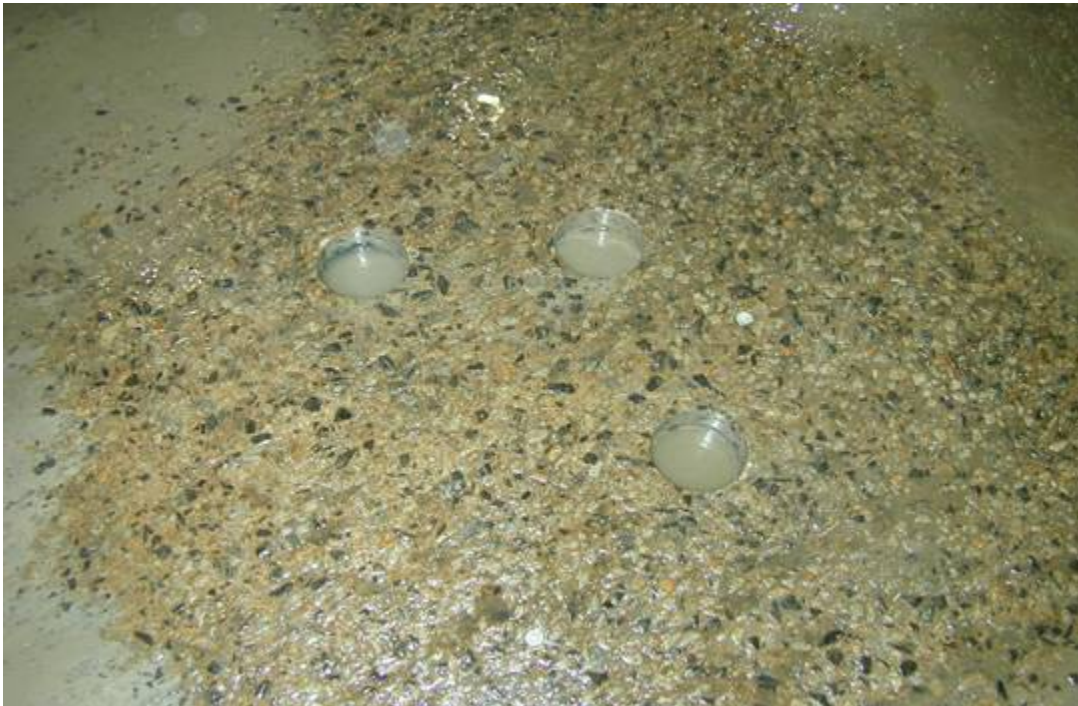
Figure 3: Close up view of the treated and untreated tipping floor concrete
