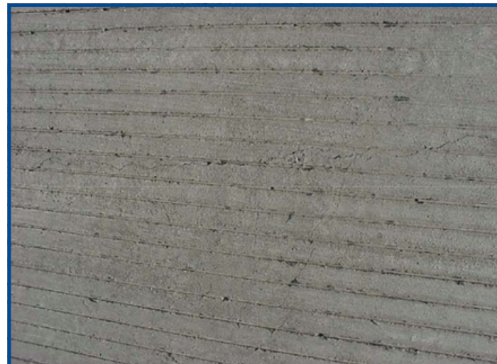
RIGHT: The Micro-cracking that is throughout the bridge deck
